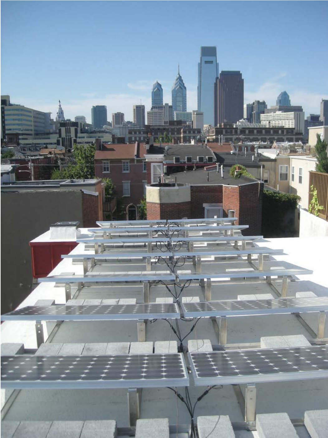
A 3kW rooftop PV was installed in the Center City District of Philadelphia. (Mercury Solar Solutions/PIX18063)
