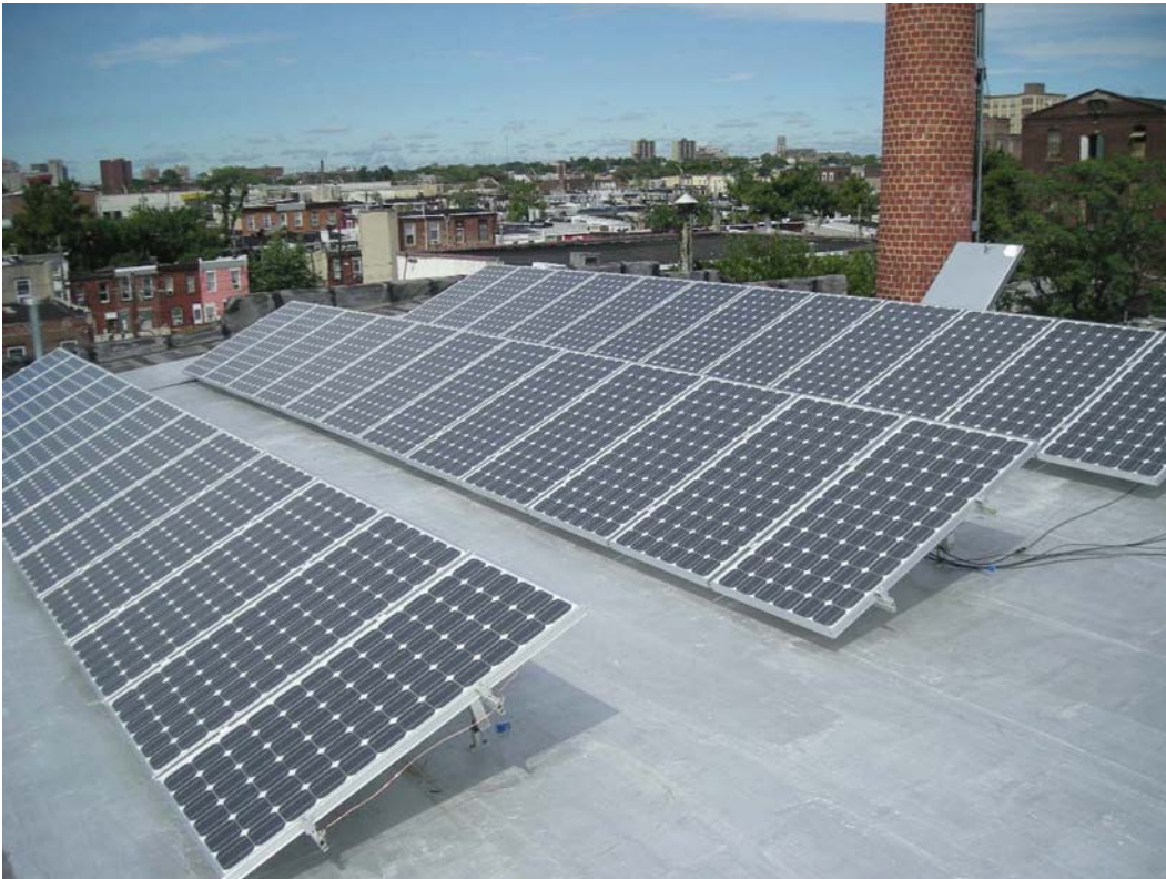
Mercury Solar Systems installed this 6 kW installation in the Lower Kensington neighborhood of Philadelphia. (Mercury Solar Systems/PIX18065)
